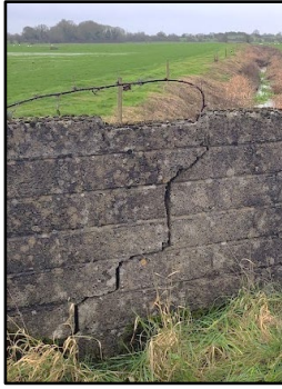
Photo 16: Settlement crack on SE parapet.
